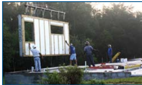
Pictured is the first wall section being lowered into place on June 24 th .
